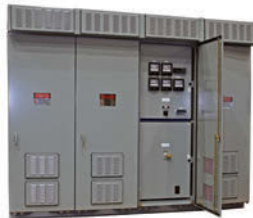
Medium voltage AC switchgear
